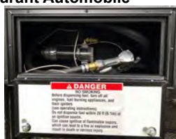
Station de Carburant
