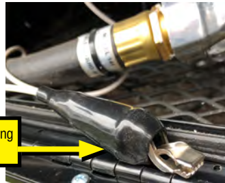
Grounding Clip Inside Fuel Station
